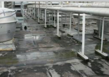
FAILING BOOTS AND FLASHING
